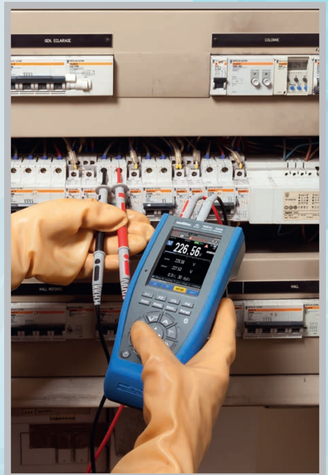
Measurements on electrical cabinets
